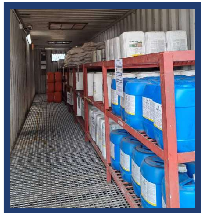
The storage and handling of herbicides at Kilombero shows good practice with secure containerised storage, non-absorbent materials and spill mitigation system in place.
