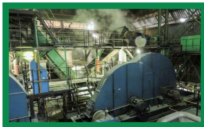
Generator room in Dwangwa
